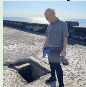
Hazards to avoid
